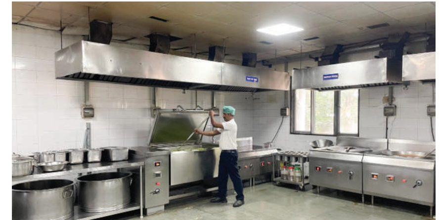
Electric Steam Induction system at Mahindra City canteen
