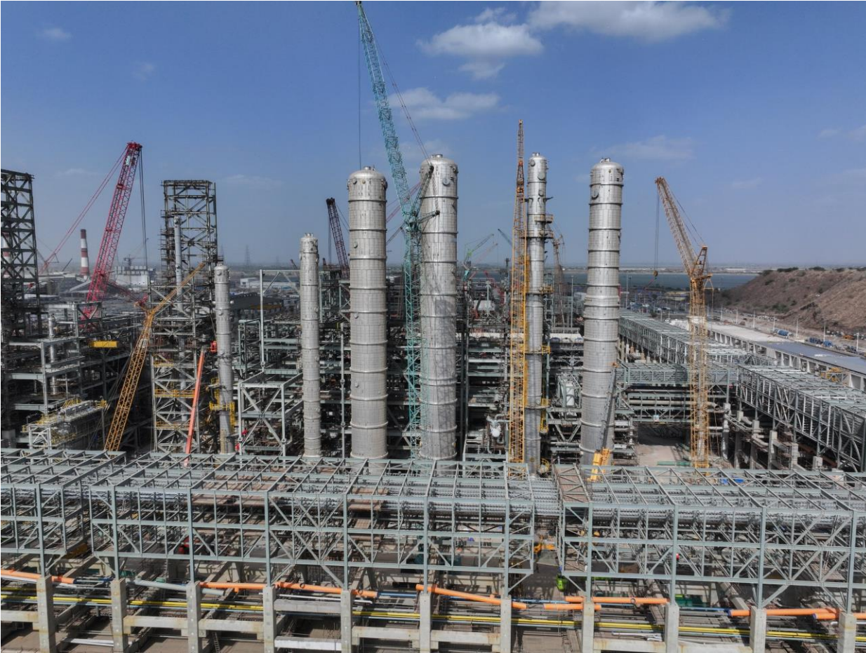
Hydrochlorination Distillation Columns
