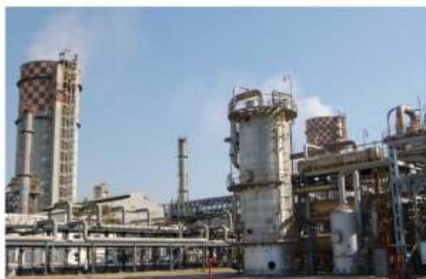
VIJAIPUR I & II PLANT
