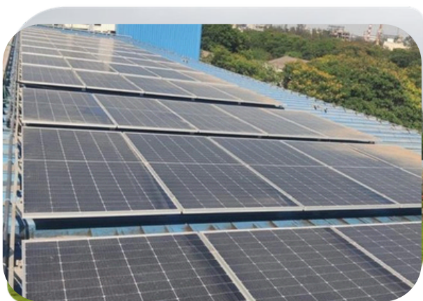
Rooftop solar panels - Ankleshwar Plant
