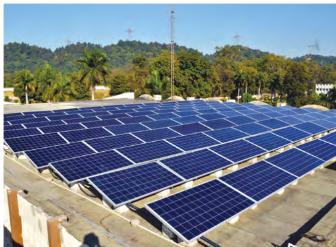
5MW Solar Power Plant at HEEP, Haridwar
