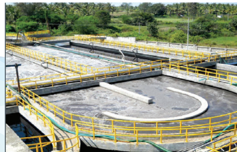
Effluent Treatment Plant – Bioconserve Renewables Envirotech, India (Subsidiary of Batliboi Ltd.)
