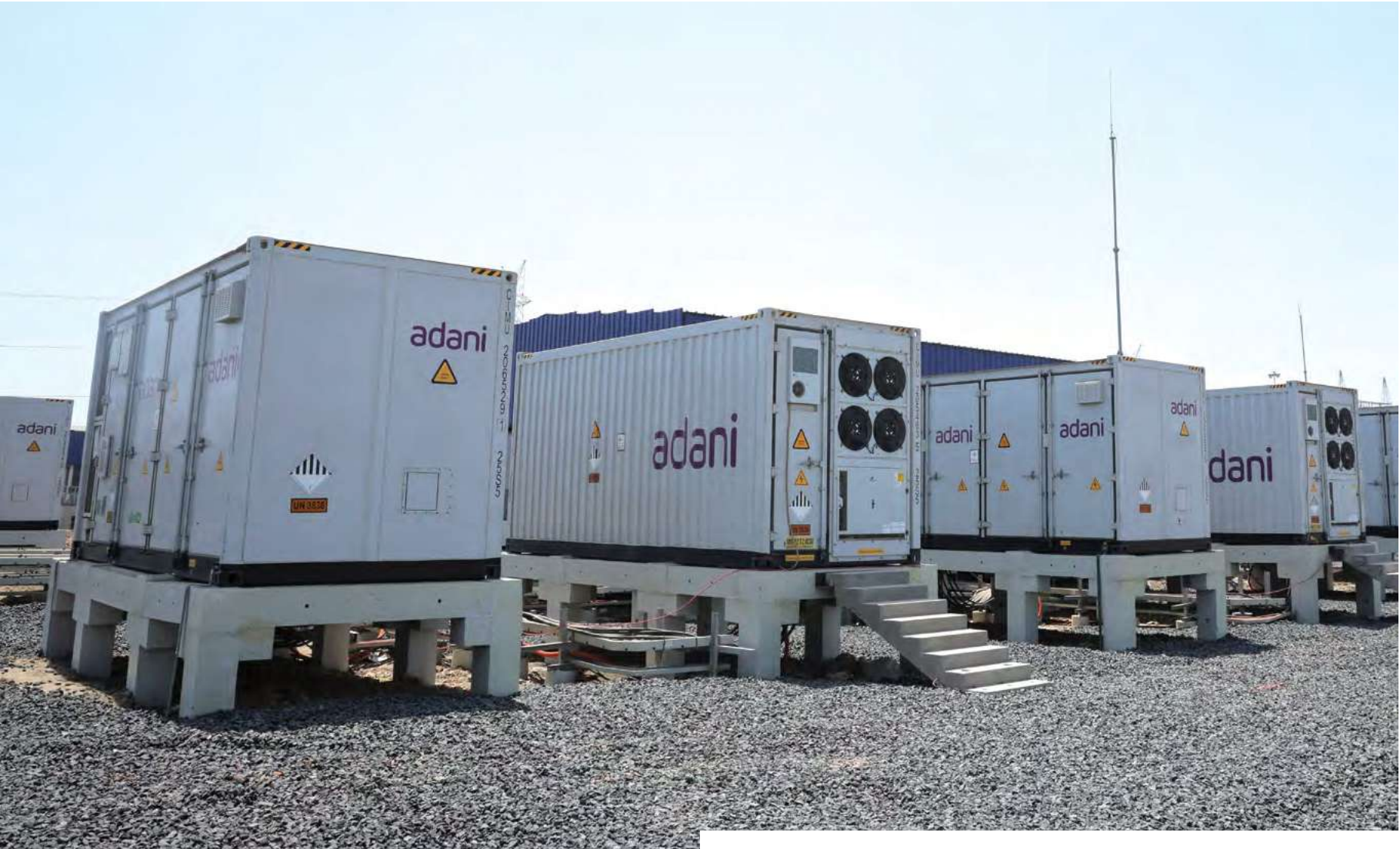
World's largest single-location Battery Energy Storage System outside China
